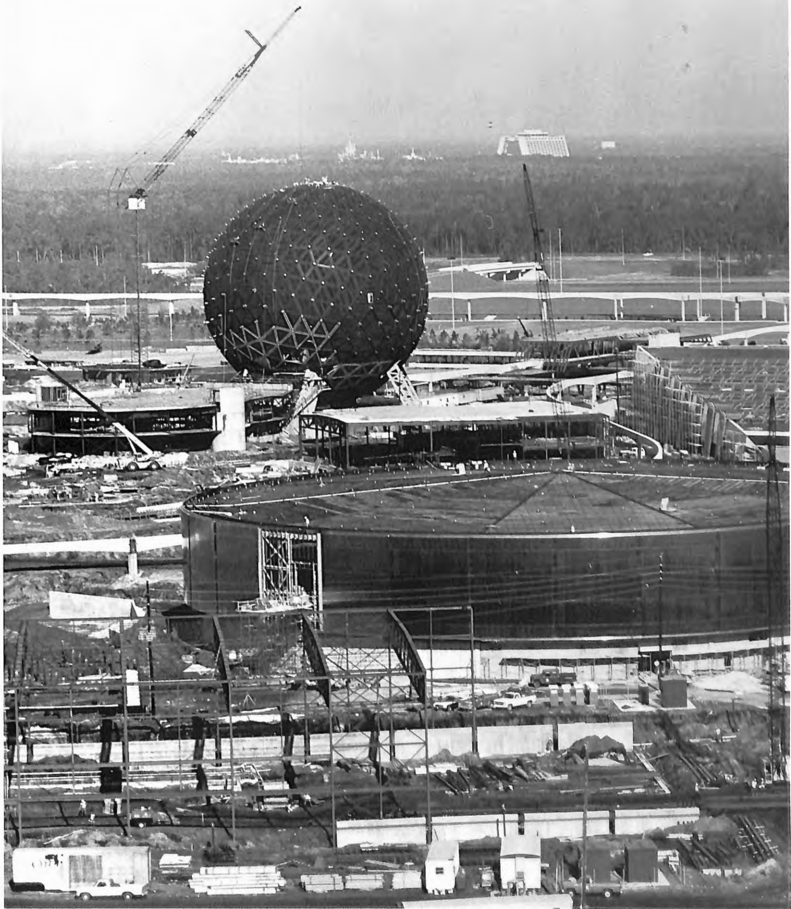
Construction continues on Central Florida's newest attraction. The three pavilions pictured in future world are: World of motion (foreground), the Universe of Energy (right), and Spaceship Earth (left).
