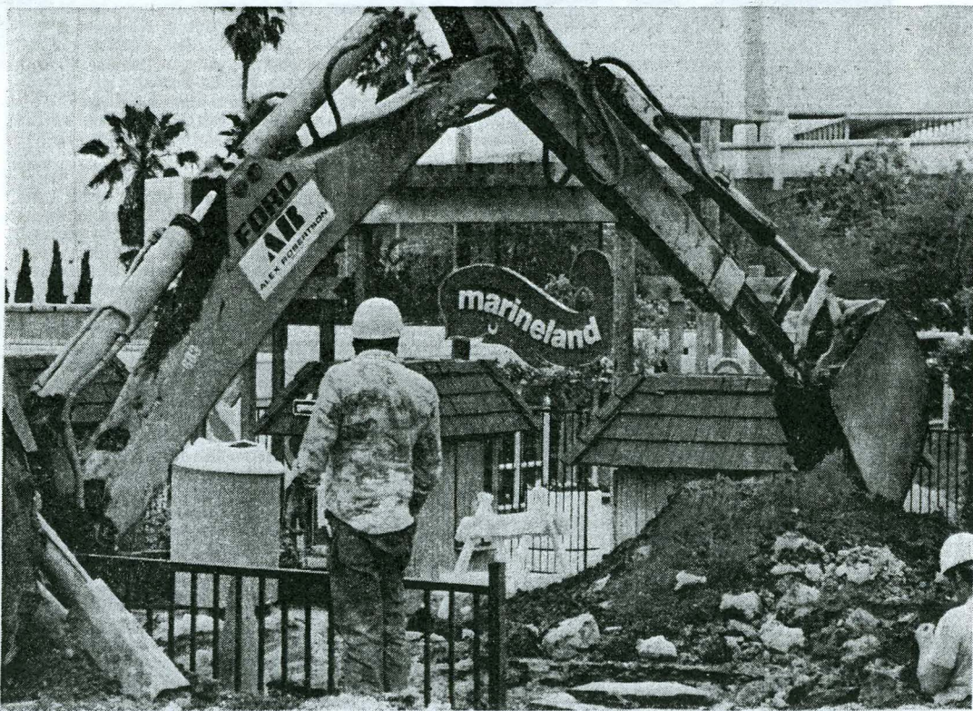
FACELIFT FOR MARINELAND —Large backhoe digs up front entrance to Marineland in major refurbishing of park. Taft Broadcasting Co., which bought Marineland last fall, hopes to pump new life into attraction which has been declining for the past decade.
