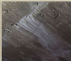
Example of efflorescence from the eastbound Seabreeze Blvd Bridge Inspection
