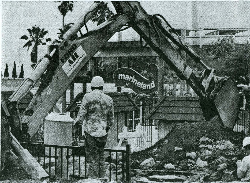
FACELIFT FOR MARINELAND —Large backhoe digs up front entrance to Marineland in major refurbishing of park. Taft Broad-
