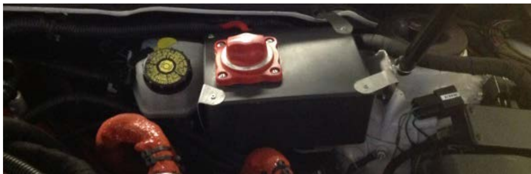
Figure 61: New 12V Distribution
