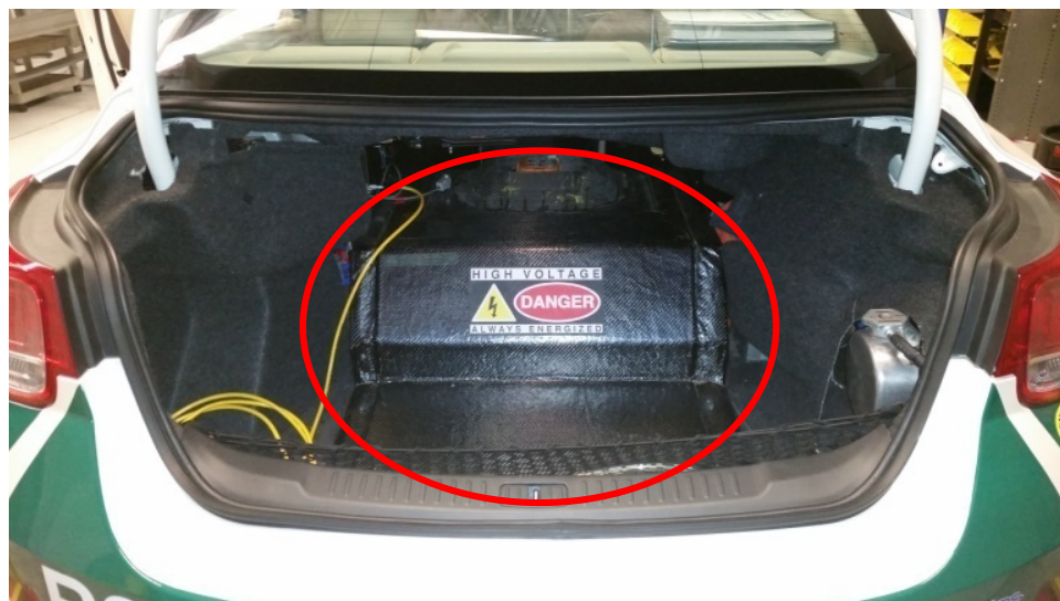
Figure 3: ESS Battery Pack
