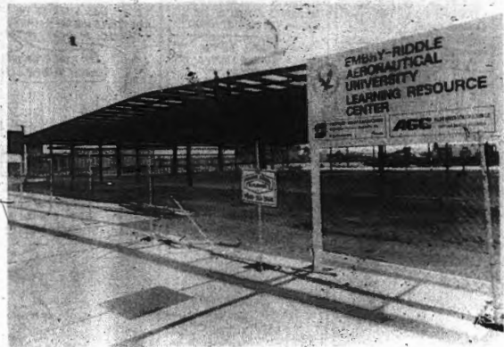
Construction of the new Learning Resource Center is progressing on schedule in the
