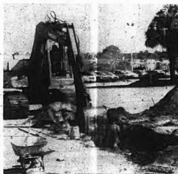
Equipment operators work to build a storm drain from the library area to the drainage ditch on the east side of campus.
