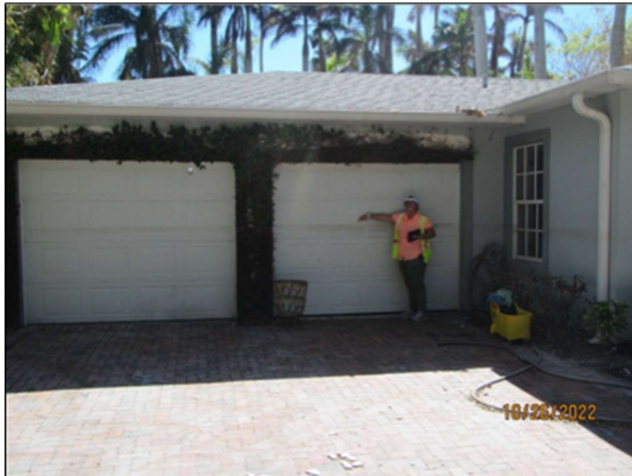
Figure 11 shows a Florida Department of Environmental Protection (2022) employee indicating the approximate height of a stain line left by Hurricane Ian in Naples, FL. Note the roughly 1/2 foot width of the stain line; this broadness results in ambiguity of measurement, and High Water Marks are therefore regarded as only marginally reliable for validation purposes.
