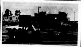
Light poles were brought to the campus, and installed in the new parking lot during the weekend. This marked the completion of this new facility.
