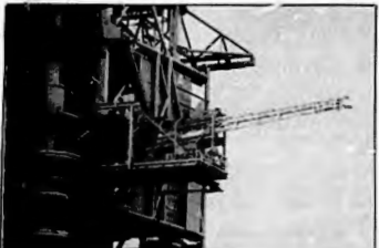
Space age junk... Workers at the Cape have removed two Shuttle/Centaur rolling beams from the fixed service structures at Complex 39. The beams were built to load liquid hydrogen into an upper stage inside an orbiter. At lift off, a 15,000-pound counterweight would drop, pulling the beam away as the Shuttle launched. Safety problems forced the cancellation of the Shuttle/Centaur program in 1986. The beam pictured is from Pad B and extended in the loading position.
