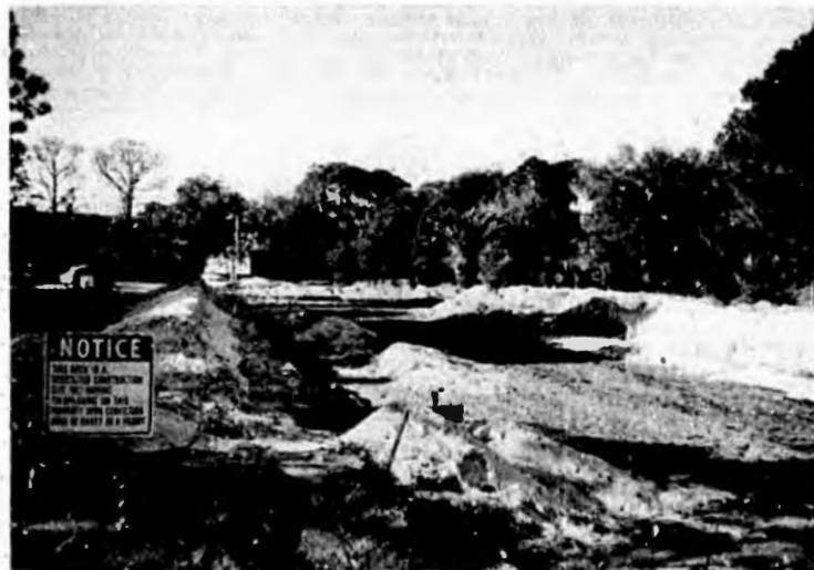
Construction has begun on the Data Processing facility located between Dorm 1 and Clyde
