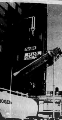
The last Atlas-Centaur is removed from launch pad 38-B following a work platform accident on July 13, 1987.
