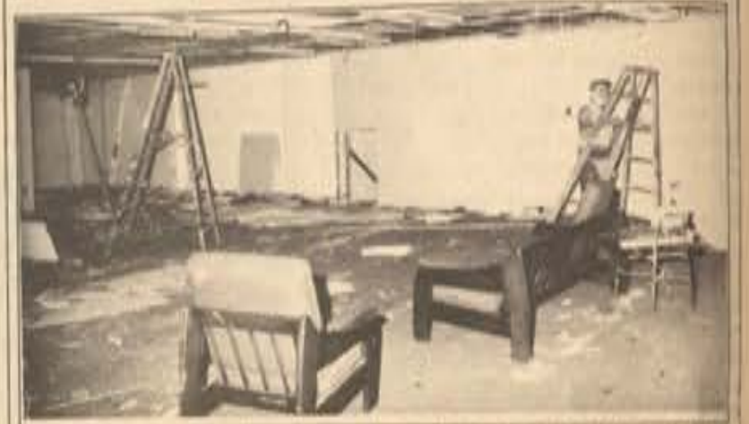
The Career Center is undergoing construction which should be completed before the beginning of this fall.
