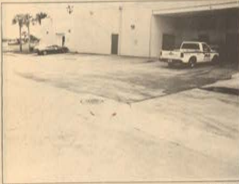
Messy... It required six hundred pounds of absorbent material to soak up the hydraulic spill that was left unattended for hours last Thursday. A stain on the pavement is all that remains.
