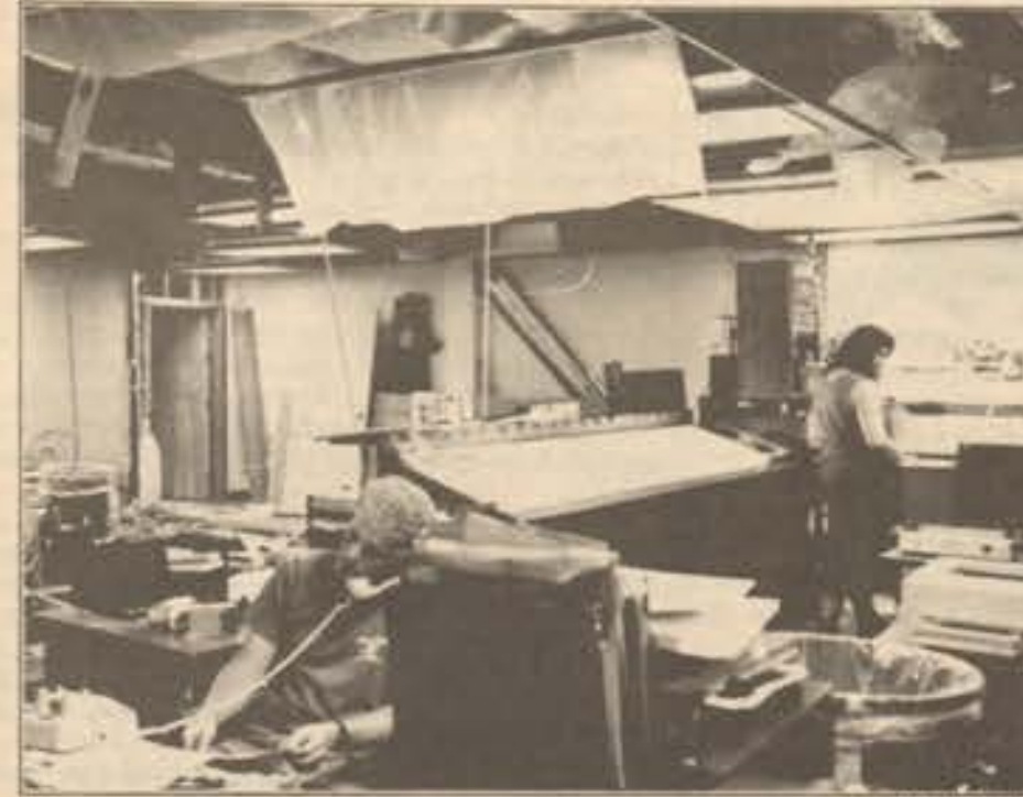
The old Avion office pictured here in a state of demolition has since been fully renovated.
