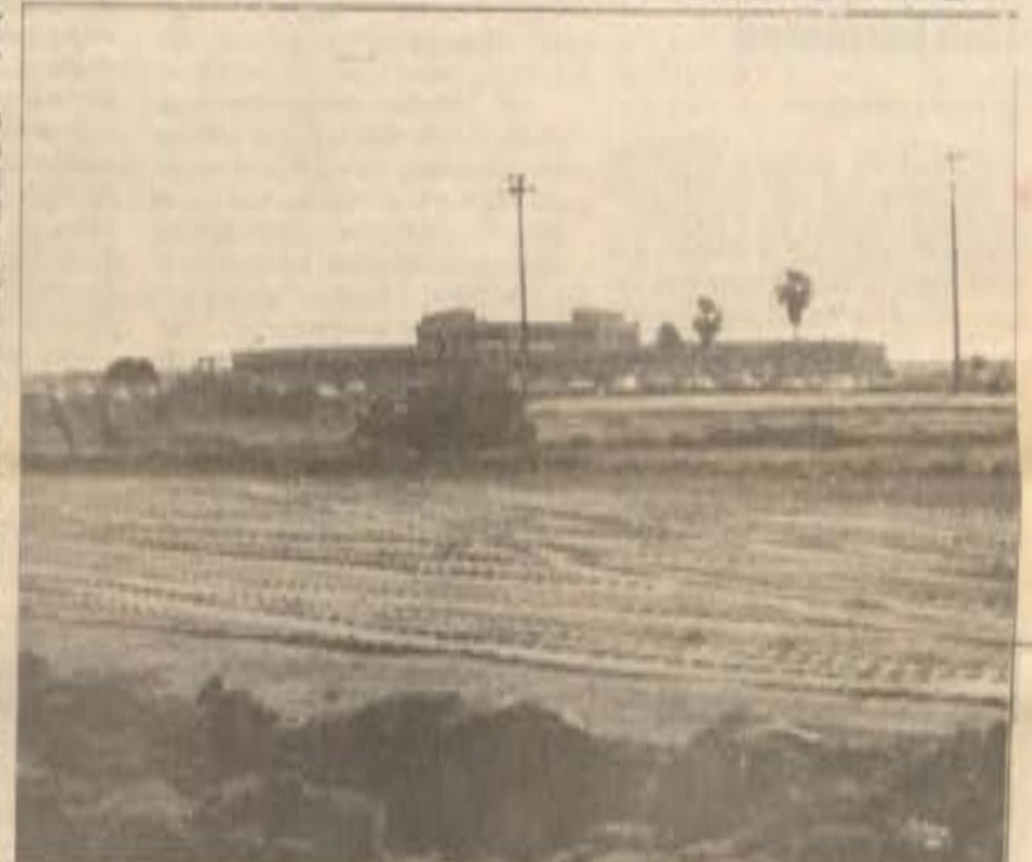
Facelift... Renovations to end drainage problems that have plagued the softball field are progressing.
