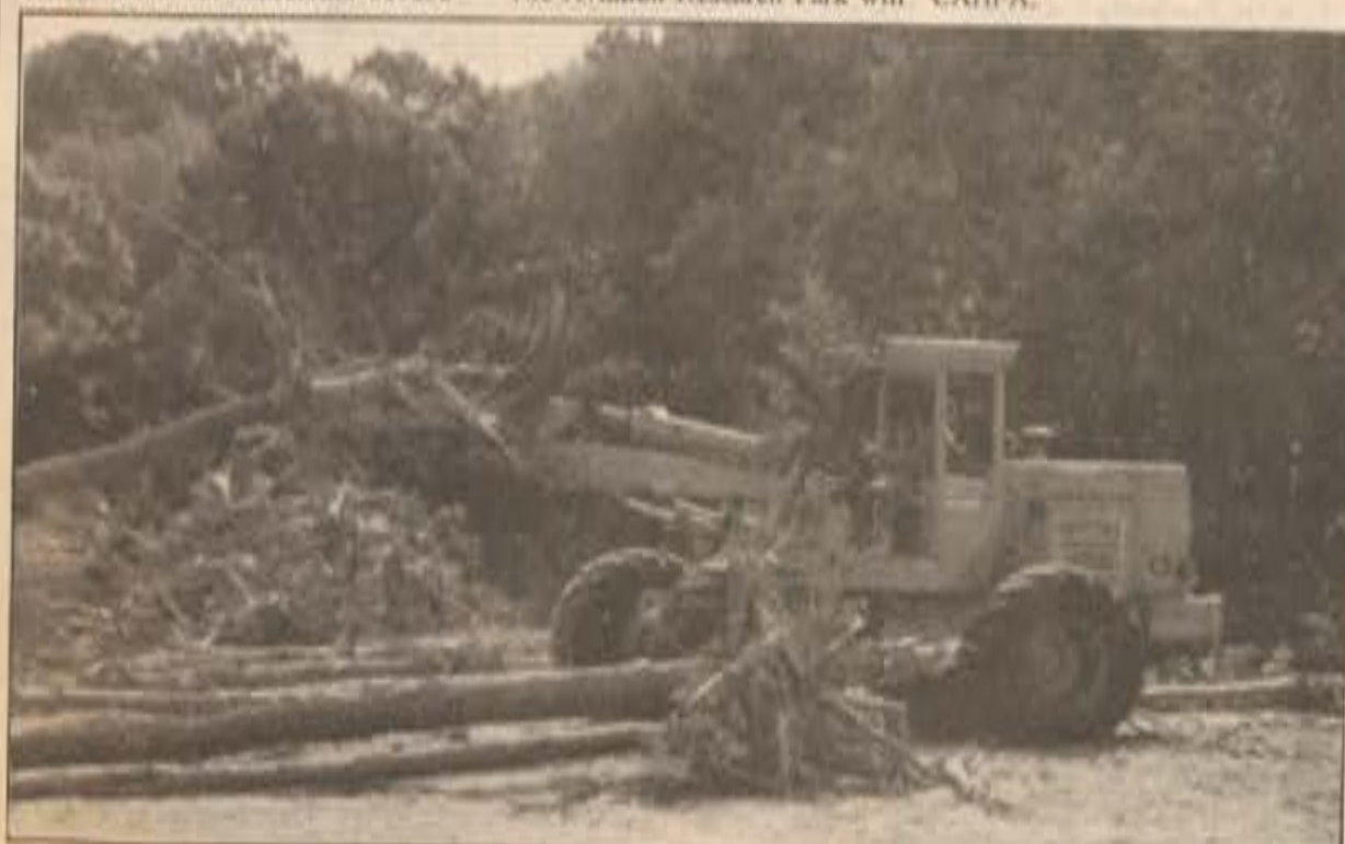
Heavy equipment from D&W Paving is excavating behind the ASSL in order to put in a new parking lot. The parking lot is designed to facilitate up to six new buildings.
