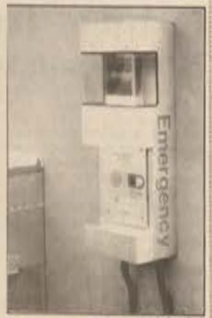
The Safety Department hopes that emergency phones like this will increase safety on campus.
