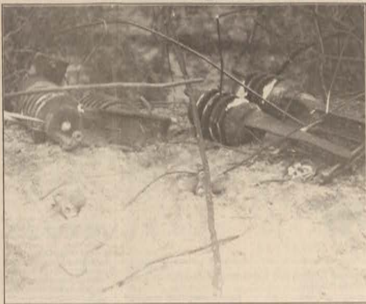
Burnt transformers attest to the severity of the fire. Residents were without power while FPL workers feverishly attempted to restore power to the area.
