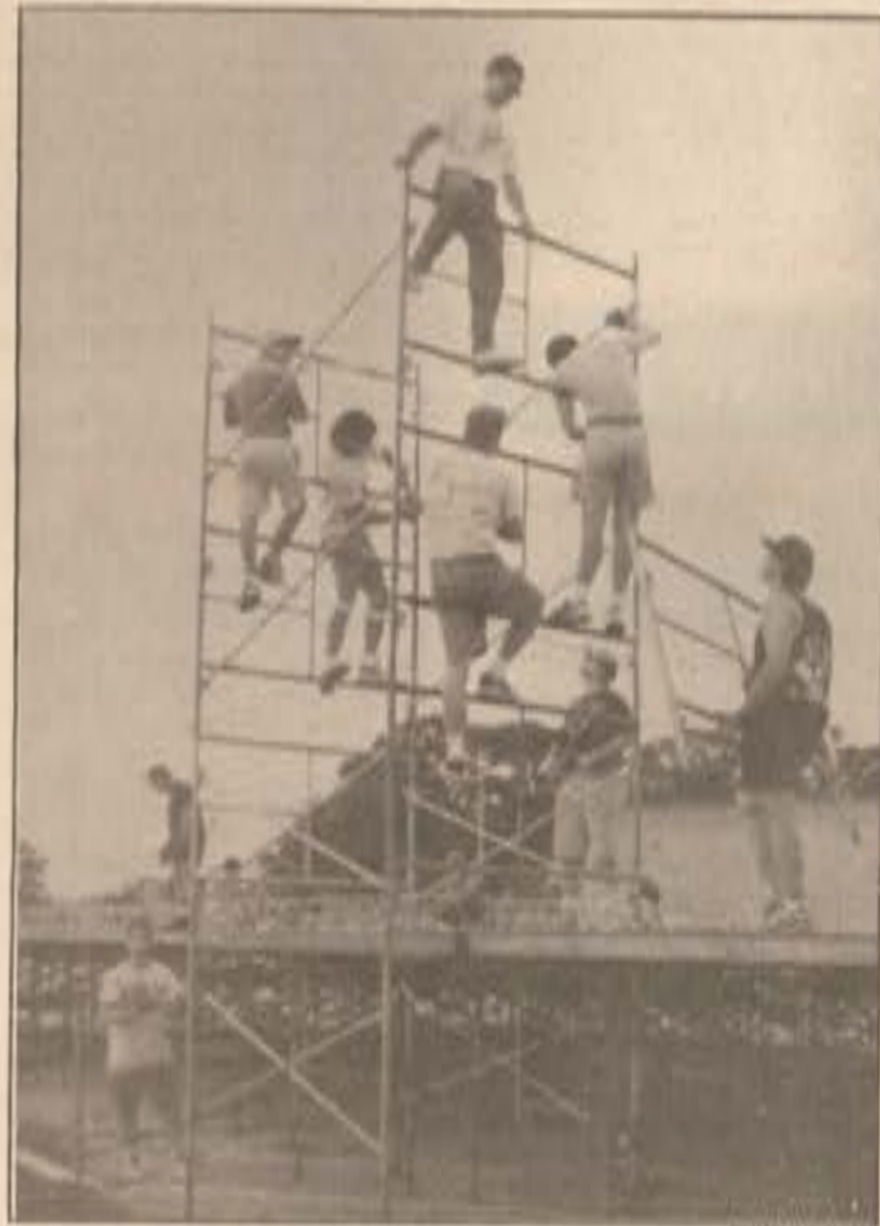
STUDENT CREWS BEGIN RAISING the framework for the new Engineering and Technology Building.
