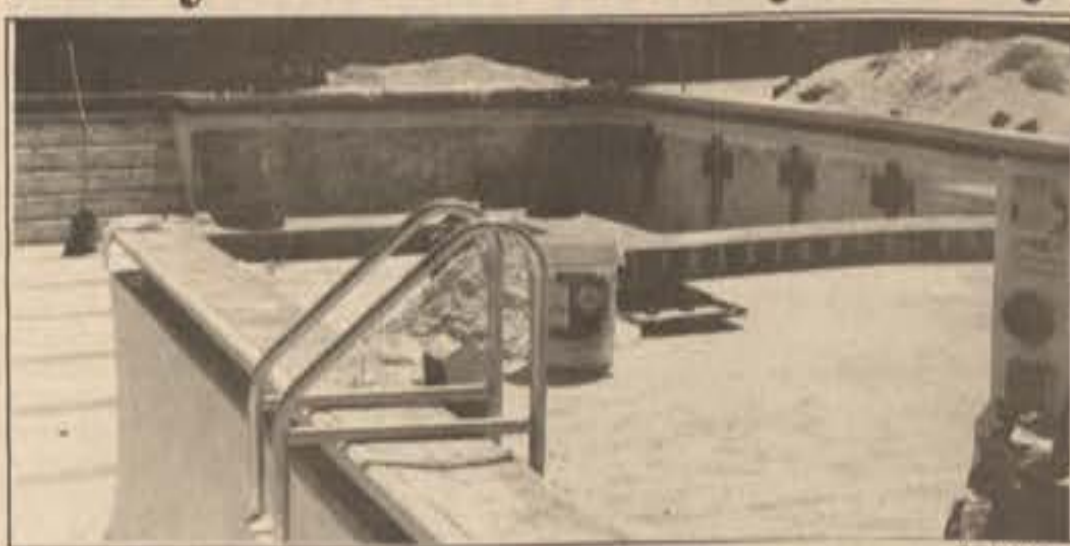
The Physical Plant performs maintenance throughout the campus to include re-enforcing the Tine W. Davis swimming pool and sodding the soccer fields.
