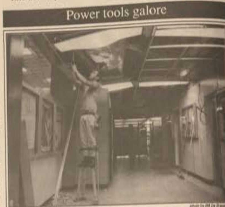
Timothy Ramsey, a construction worker, is using stilts to install new wiring in the Student Center. Ramsey and his co-workers are also installing new acoustical tiles, air conditioning ducts, and light fixtures. This is all part of the general upkeep of the building.
